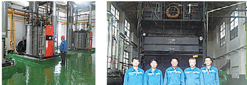
本集團最後一家煤改氣工廠 — 湖南工廠淘汰燃煤後嶄新的燃氣鍋爐房。 The new gas boiler installed after elimination of the coal-fired boiler in Hunan factory, the last coal-to-gas plant of the Group.
