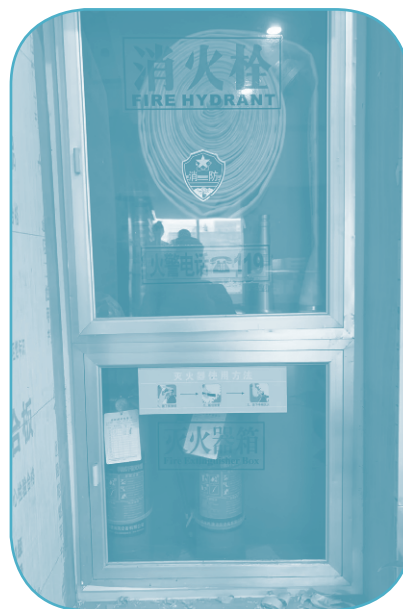
Firefighting equipment is installed in our office.
